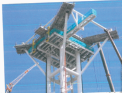
Pyeroy scaffolding used on the new 1,250 metric ton (1,378 ton) Seabrover being built for Centrica by Heerema Fabrication Group in Hartlepool.
